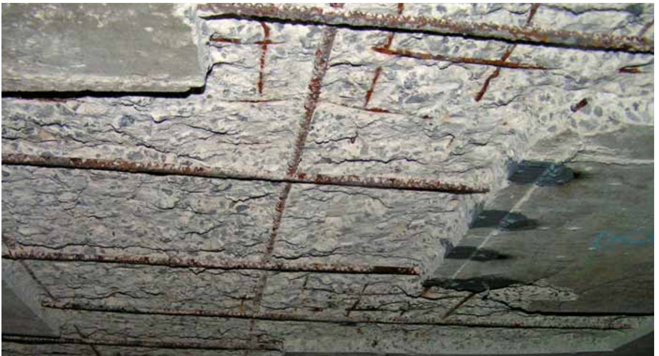
Figure 2: Example of spalling and cracking due to concrete corrosion.
