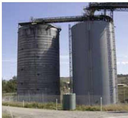
Figure 2: This before-and-after photo shows the silo on the left awaiting repair, while repair to the silo on the right had just been completed.
