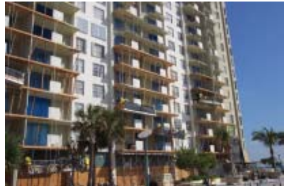
A new CP system is being installed on the balconies of Miami Beach's Roney Palace hotel and condominium complex. Photo courtesy of MATCOR, Inc.
