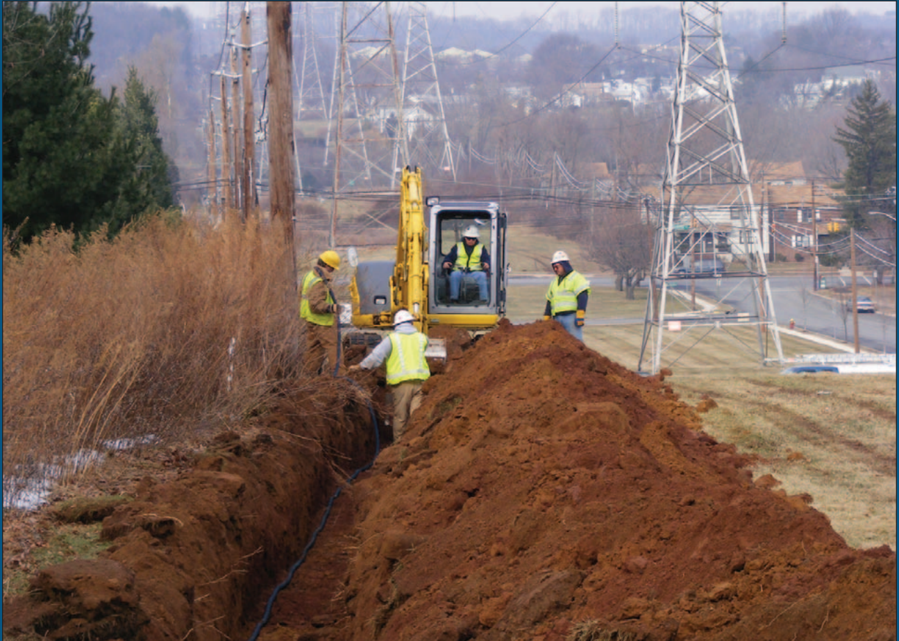
The new induced AC mitigation system is installed along Williams Gas Pipeline's Transco system, which lies along a HVAC corridor in northern New Jersey.
