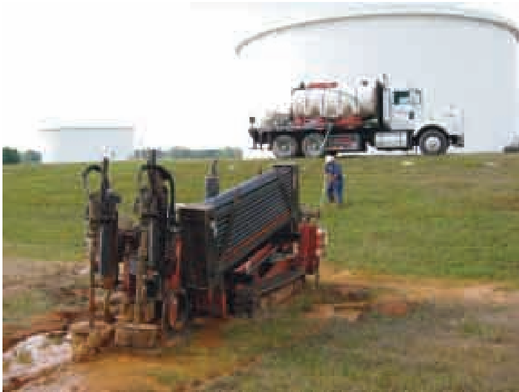
Horizontal directional drilling under an existing AST to install a leak detection tube and reference electrode assembly rings prior to backfilling
