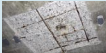
Before: An actual roof section demonstrates the rebar corrosion prior to installation of the MATCOR CP system.
