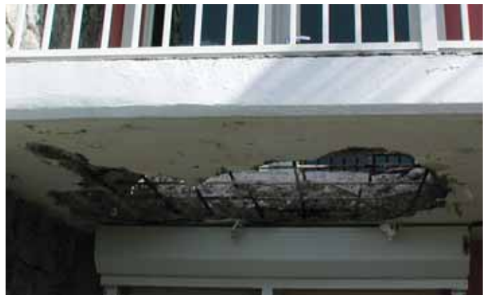
Corrosion of the rebar in concrete balconies, bridge decks, and swimming pools is a significant problem along the Florida coast. MATCOR's enhanced website has a tutorial on the causes of corrosion and cathodic protection, as well as the economics of the system that can help engineers explain the process to clients.
