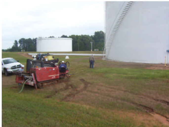
Figure 1 – Horizontal Directional Drilling under an existing AST tank to install leak detection tube and reference electrode assembly
