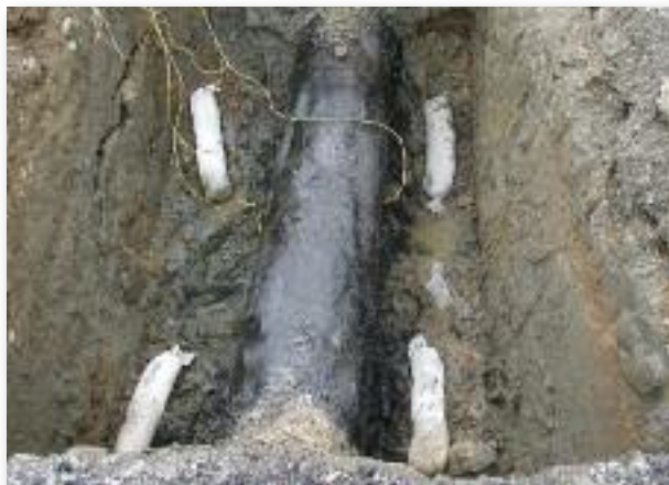
Magnesium anodes were installed along the buried piping as a preventive measure and to supplement the existing CP system.
