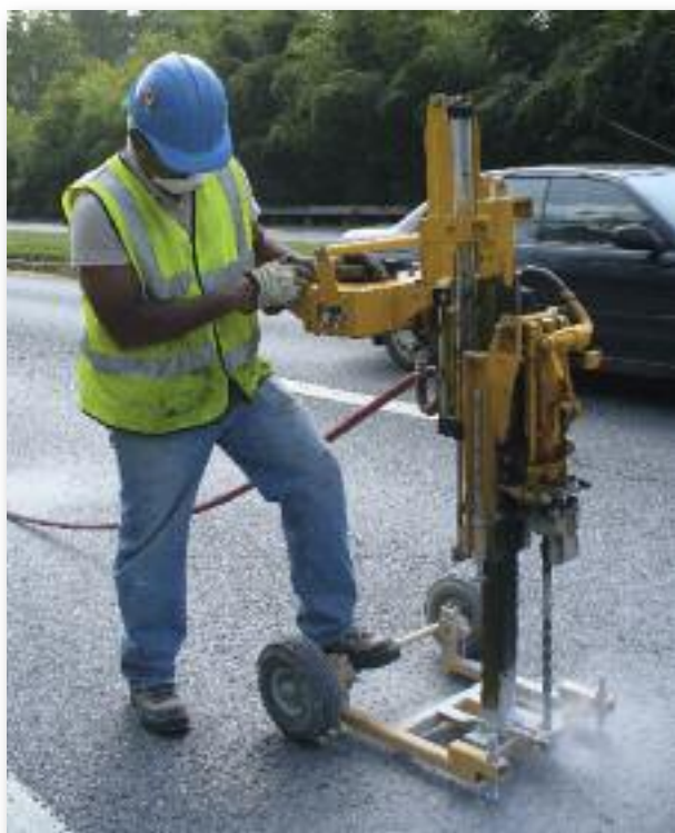
MATCOR made 1,550 holes in the road during the course of the ECDA.
