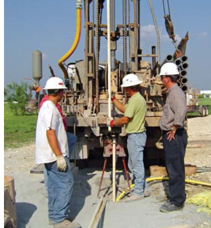
Figure 3: Recent installation of a self-contained anode system in Dallas, TX.
