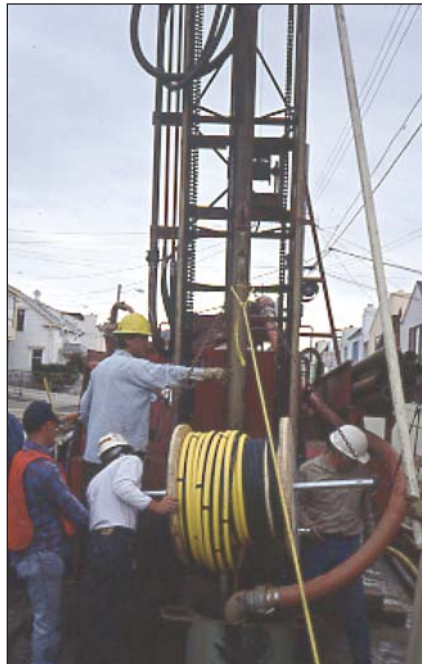
Figure 1: A self-contained anode assembly being prepared for installation down-hole in a residential neighborhood.
