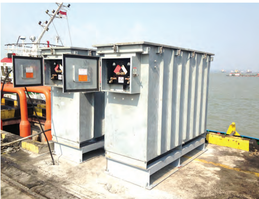
FIGURE 3 CP system rectifiers.
