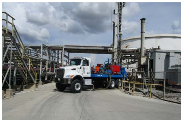
Figure 1. Vertical drill rig used to install deep anode systems in a vertically drilled hole, typically to depths of 50 – 150+ m.
