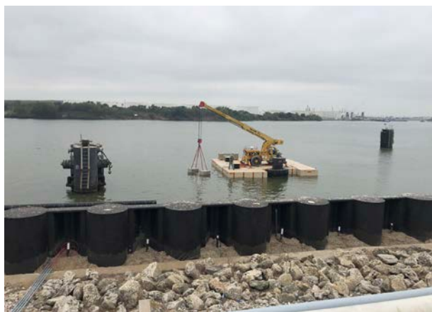
Figure 2. Sled Anode Assembly being installed in the channel using a barge mounted crane to protect the combi-wall in the foreground.
