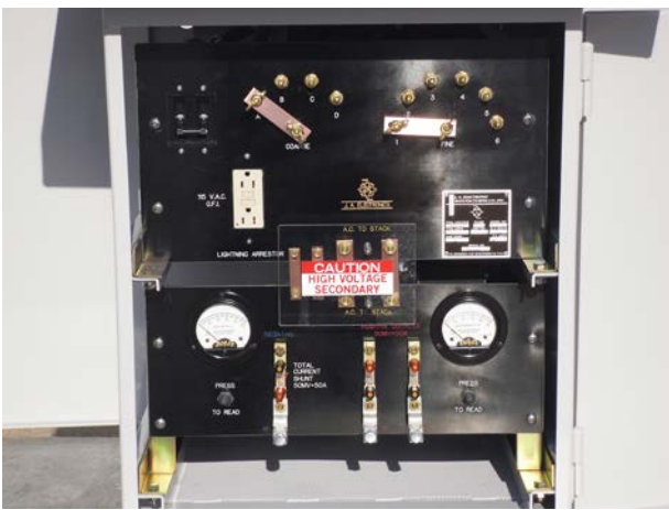
Figure 2. Typical air cooled rectifier – impressed current CP system DC power supply.
