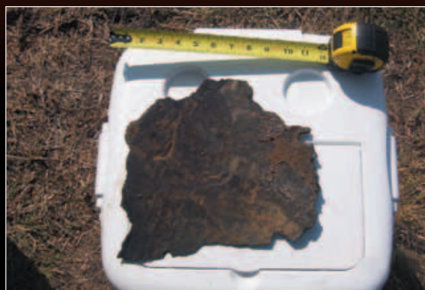
Figure 1. Coal tar enamel coating disbonded from pipeline. This sample was located close to the system rectifier.
