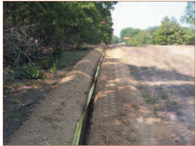
Figure 4. Linear anode installation complete with warning marker tape immediately prior to backfill.
